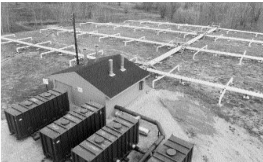
The volatilization system that removed dangerous organic compounds that contaminated ground water around the Twin Cities Ammunition Plant, Minn.
