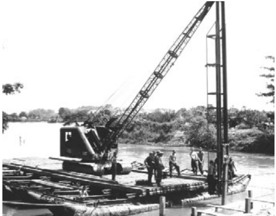
Soldiers of the 1st Engineer Battalion driving pile for the construction of a new bridge near Di An
