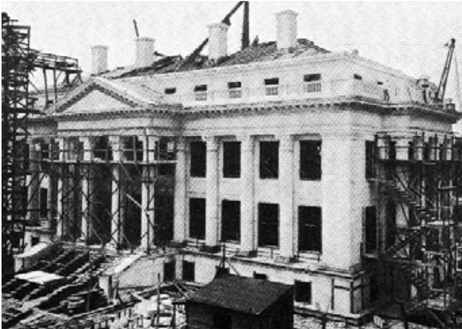
Red Cross Building built as a memorial to women in the Civil War, under construction, 1916
