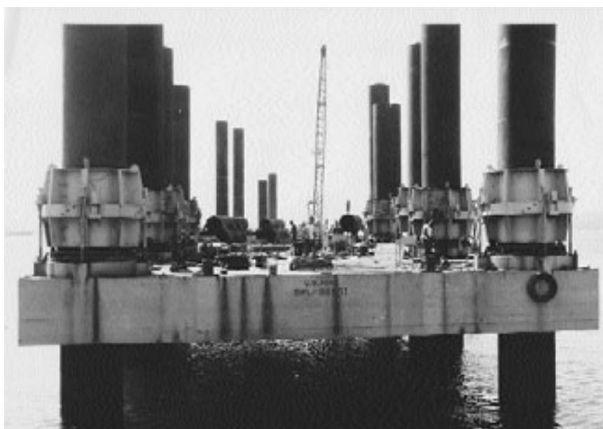
DeLong pier floated into position with caissons ready to be driven down, Cam Ranh Bay, December 1965.
