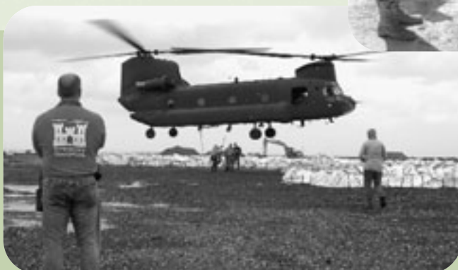
Chinook helicopter prepares to lift 5,000-pound sandbags to repair damaged flood walls.
