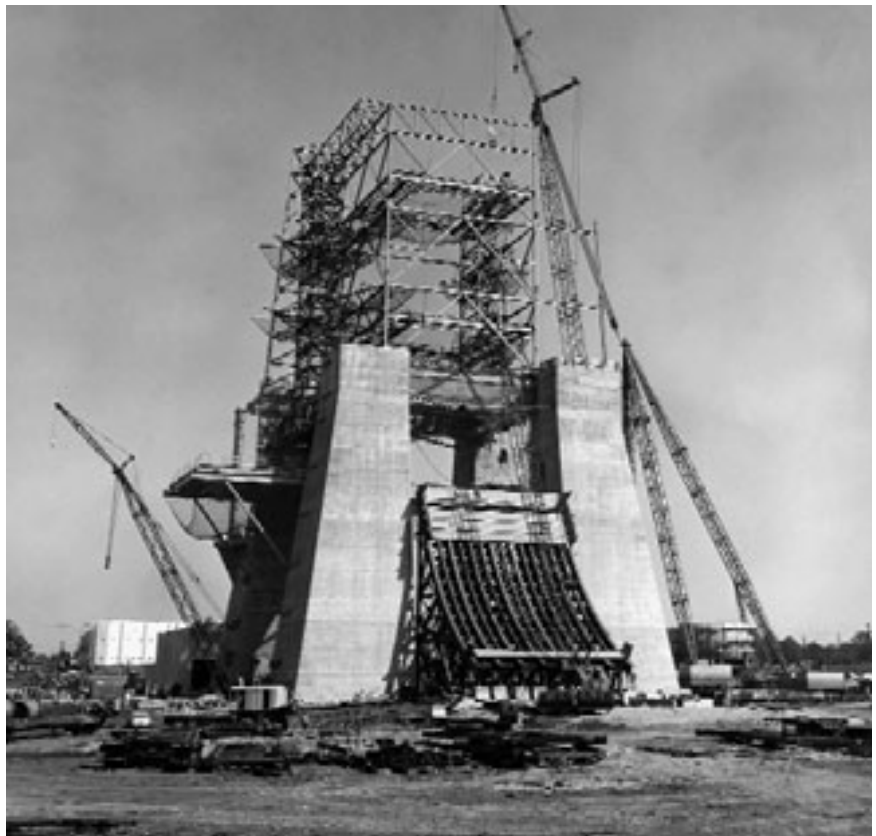
Constructed at the George C. Marshall Space Flight Center in Huntsville, Ala., the Saturn V test stand was designed to withstand 7.5 million pounds of thrust.
