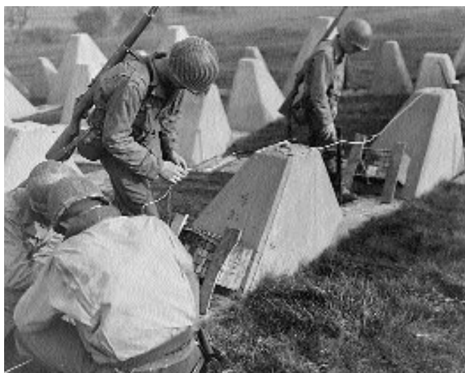
Placing explosive charges to demolish concrete tank barriers on the Siegfried Line, October 1944
