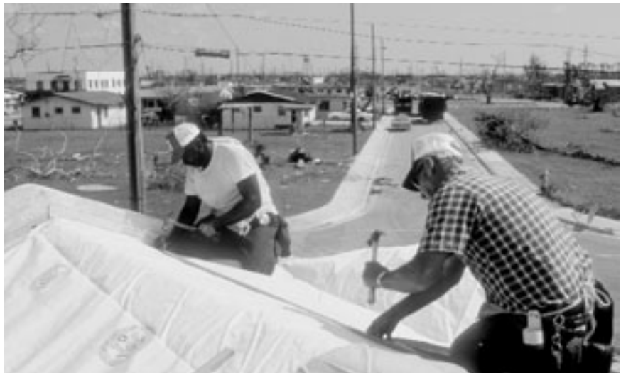
Corps of Engineers contractors install a temporary roof on a home damaged by Hurricane Andrew.
