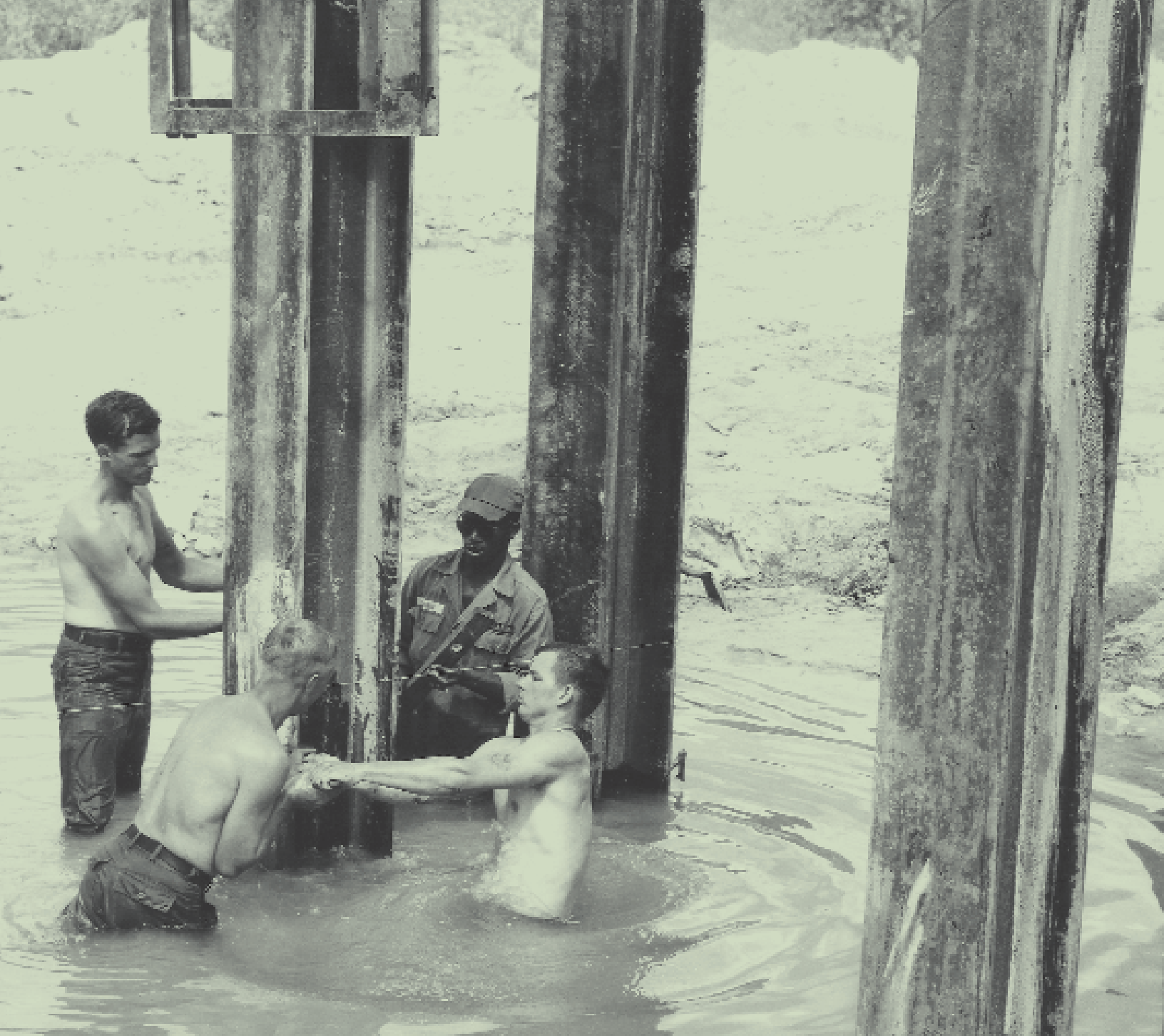
Soldiers of the 299th Engineer Battalion check the alignment of piles before they are driven, May 1966.
